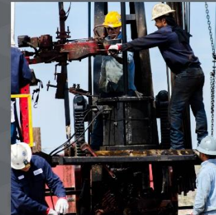
Rig Floor Tubing Systems
